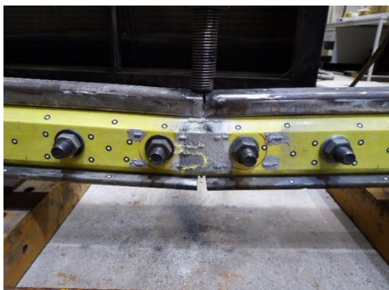
Fig. 7. Insulated rail joint with fishplate type II after 7,331 loading cycles (both fishplates damaged)
